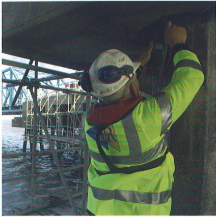
Figure 3: An engineer tests the electrical resistance of a cathode in the ICCP system at the Stena Ro-Ro terminal, Fleetwood.
