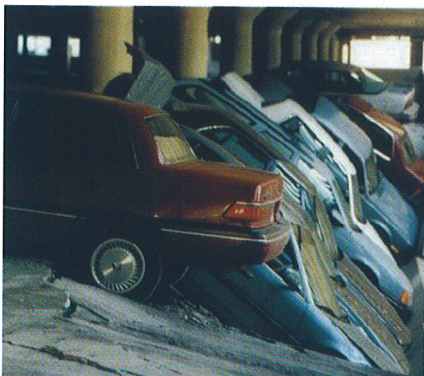
Figure 1: The MONY car park, Syracuse NY which collapsed without personal injury due to reinforcement corrosion.
