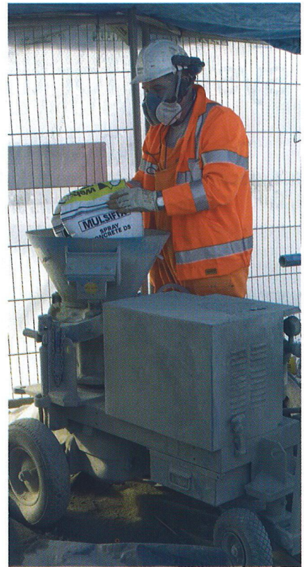
Figure 4: An operative charges the spray concrete machine for pumping to a remote application point.
